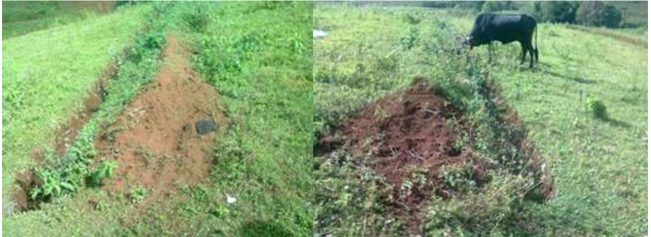
Figure 2. Weak management and maintenance practice (Cattle heard over and destroying the structure).
